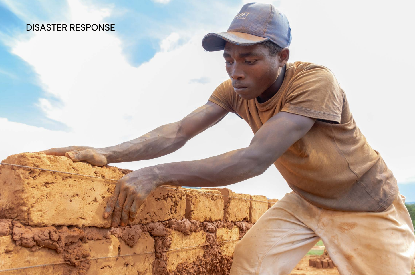
Bahati Irangunda Hakizimana, a qualified construction worker, has helped build homes for others who, like him, fled the conflict in DR Congo.
